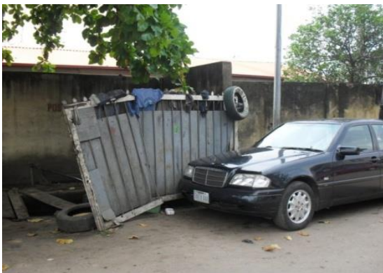
Plate 25. Surulere, Lagos photograph Source: Obiadi's field work (2015). Abandoned street gate in disrepair and serves as a stand for a community vulcanizer and motor mechanic.
