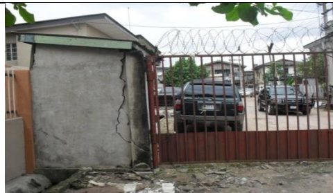
Plate 23. Surulere, Lagos photograph Source: Obiadi's field work (2015). Surulere security gate house in disrepair and abandoned for a long time.
